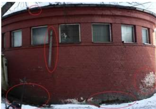
Fig.1.9 The lack of gutters, humidity on the basics
