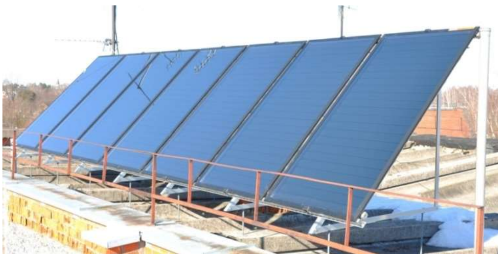
Fig.4.13. Flat solar collectors on the roof of residential building in Latvia
