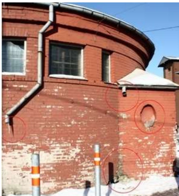
Fig.1.8 Damage to wall, the lack of guttering and window
