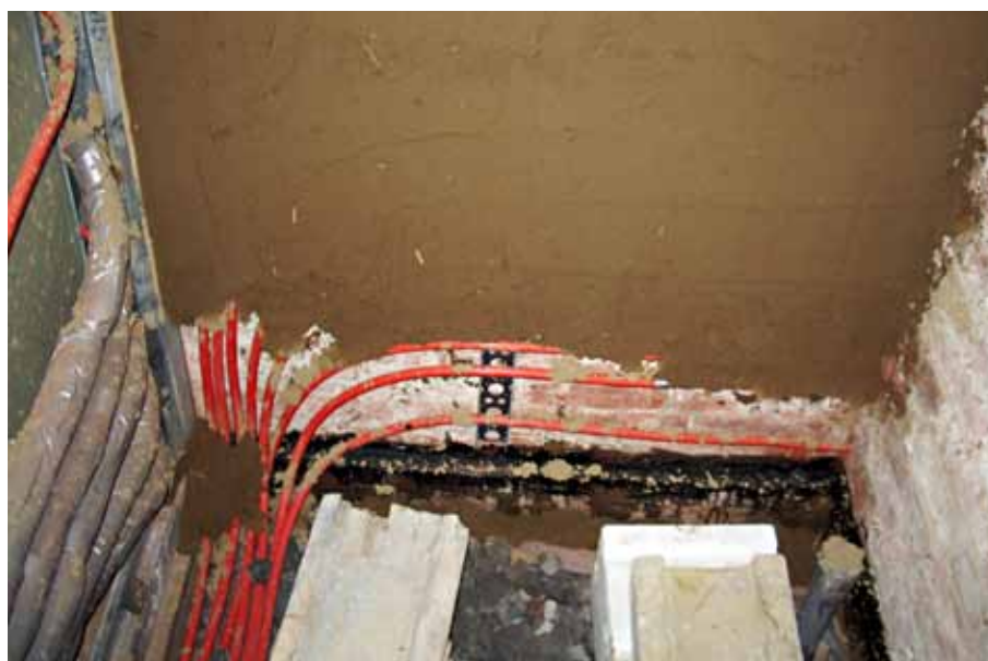
Wall tempering system, Hamburg, Germany
